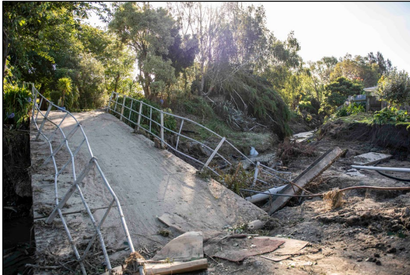
Extensive damage to roading networks has occurred across the whole region. 766
