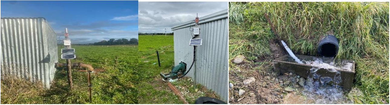
Figure 4: From left to right: Installations at O'Neils, Paddock 2 and Novaflow.
